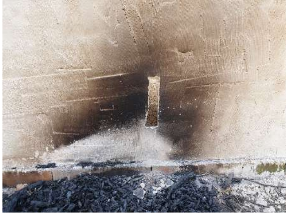
Photo 29: Site of investigation into the effect of the fire of the hempcrete located at the centre of the fire affected area
