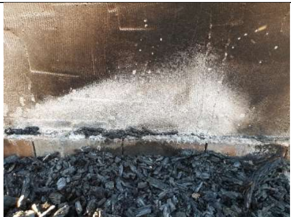
Photo 28: Close up of sound render after fire had cooled down
