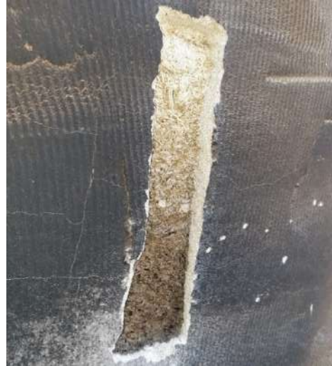
Photo 30: Condition of hempcrete beneath the render. The render thickness was 6mm at the bottom and 12mm at the top of the cut. The colour and consistency of the underlying hempcrete was not altered where the thickness of the render exceeded 9mm. with a thinner render layer some discolouration was evident
